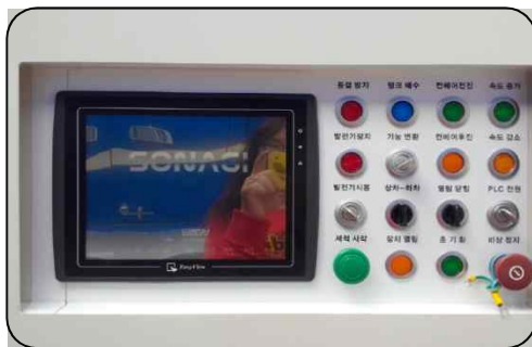
조작장치 / Monitor & control panel
